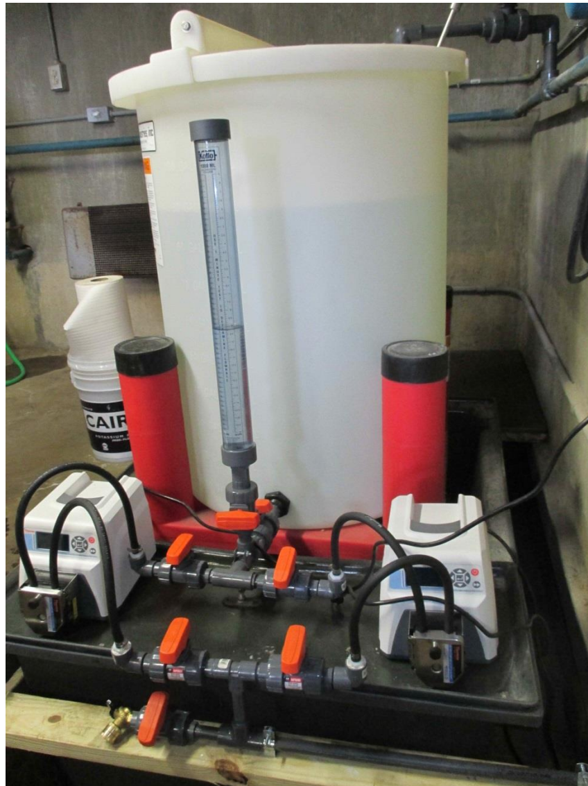
EarthTec QZ delivered to pipeline intake structure by metering pump
